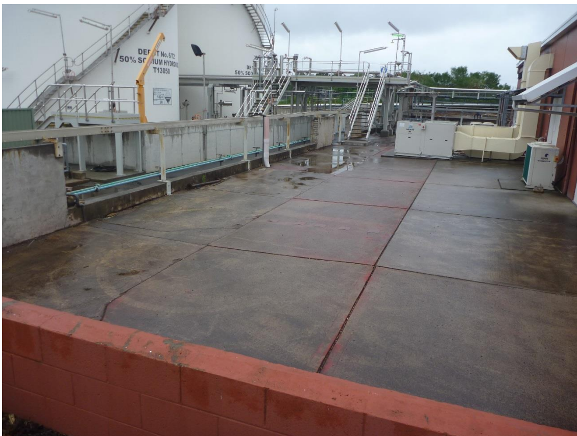
Photo 20 - Looking south-west. New MCC to be located at left. Existing control room at right.
