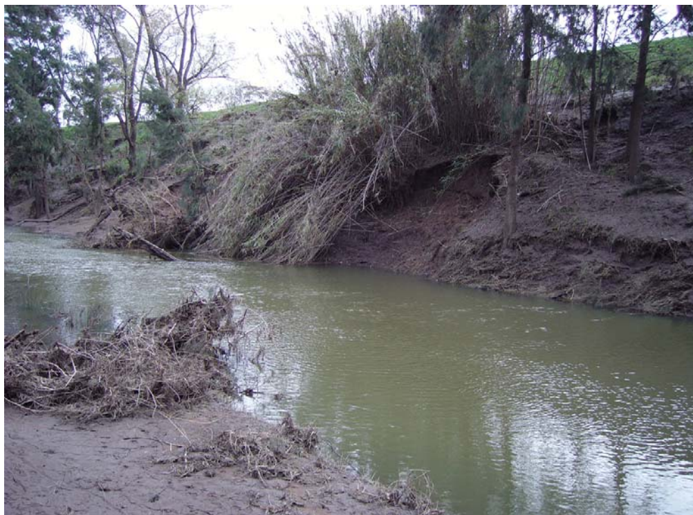
Photo 1: Riparian and in-stream scouring at the downstream
