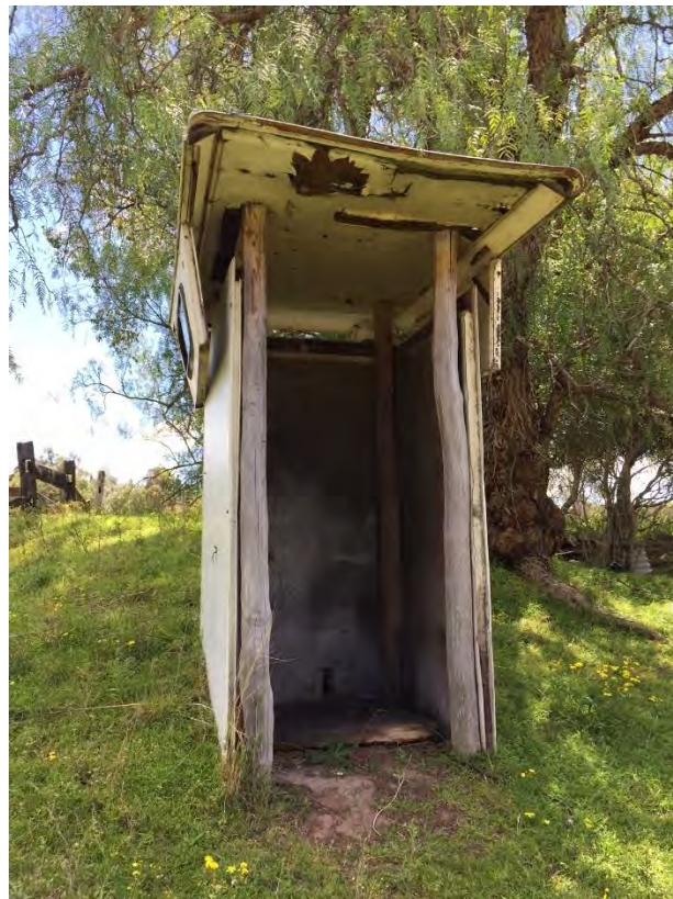
Photograph 4 – Former pump shed with fibre cement sheet walls, concrete base and dark oil staining.
