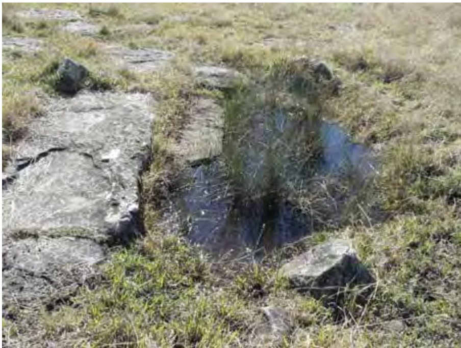
Plate 8: Jointed sandstone with trapped water in the south eastern part of the site.
