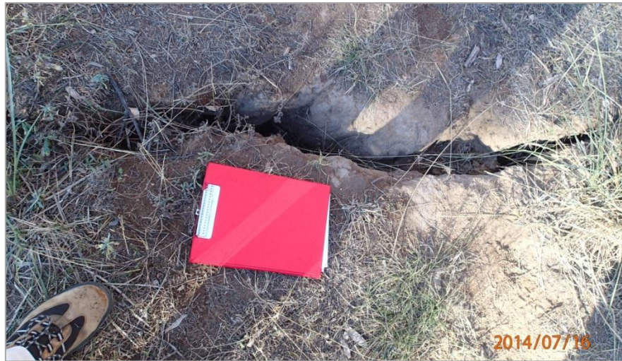
Figure 13: Example of Observed Surface Cracking near Longwall 8A
