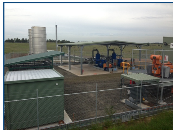
Plate 1: Typical Gas Plant
