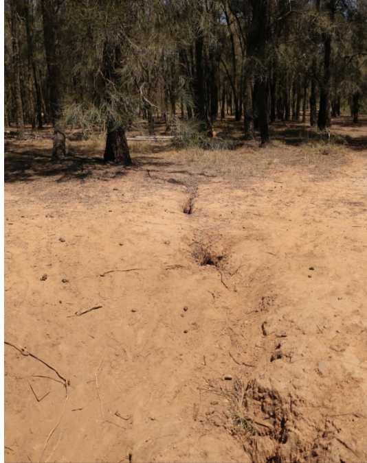
Figure 11: Crack Running Perpendicular to Bank Top Approximately 50 Centimetres Deep in Places
