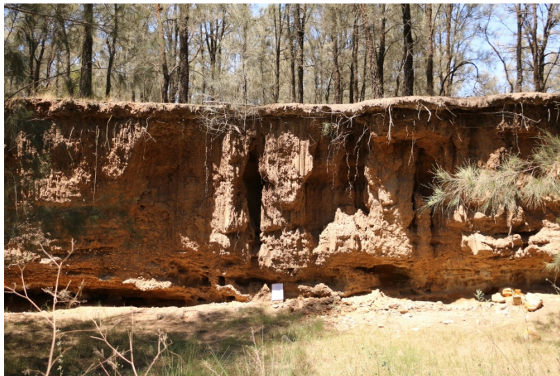
Figure 12: Vertical Eroded Banks in Sections of North Wambo Creek
