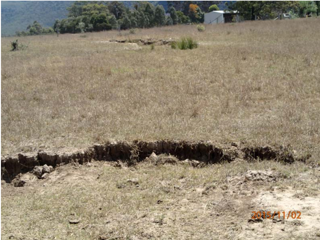
Plate 60: UW1 – Minor erosion upstream of Wambo Road
