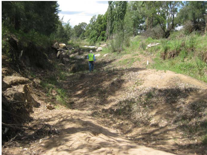
Plate 54: Wambo Creek –incised channel and eroded banks downstream of Wambo Road (looking upstream)
