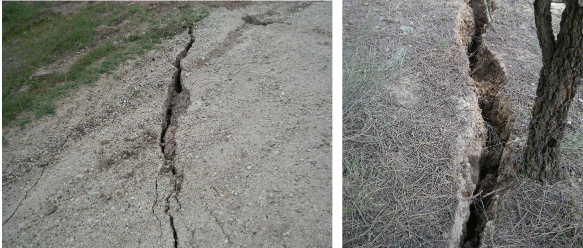
Fig. 4.7 Photographs of Surface Cracking above BSLW1 at the Blakefield South Mine
