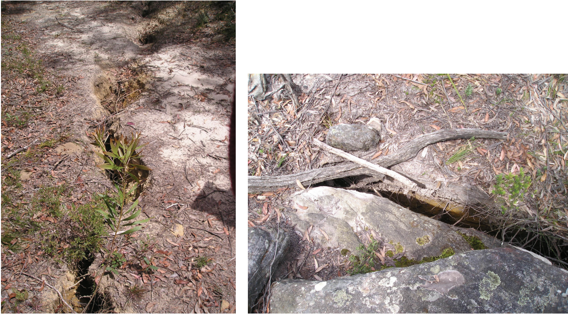
Fig. 5.25 Surface Tension Cracking due to Down Slope Movements at Dendrobium Mine
