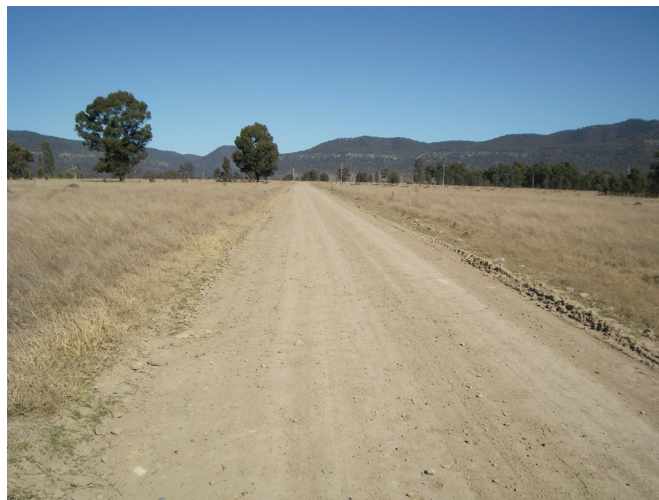
Fig. 6.1 Photograph of an Unsealed Road
