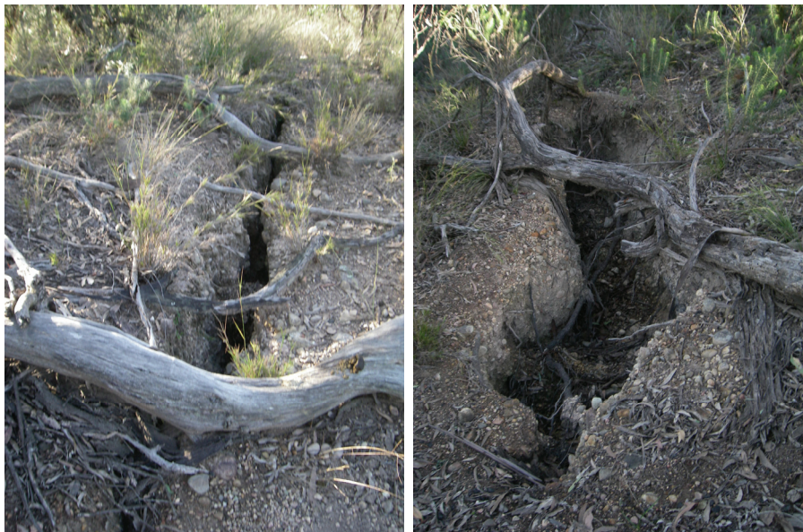
Fig. 5.23 Photograph of Surface Cracking on Steep Slopes (IMGP4101 and IMGP4102)
