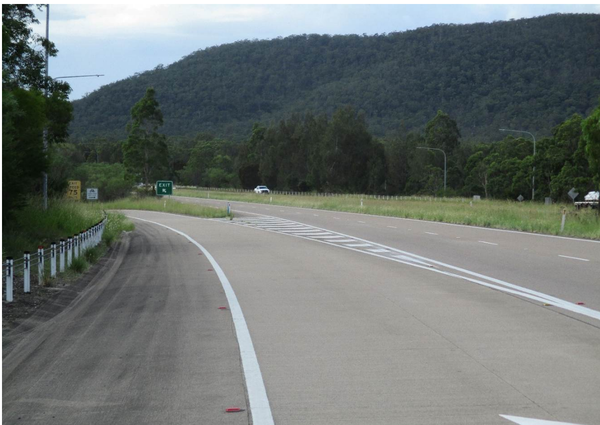
Photograph 5 – A1 Pacific Highway, Tarean Road north northbound off-ramp.
