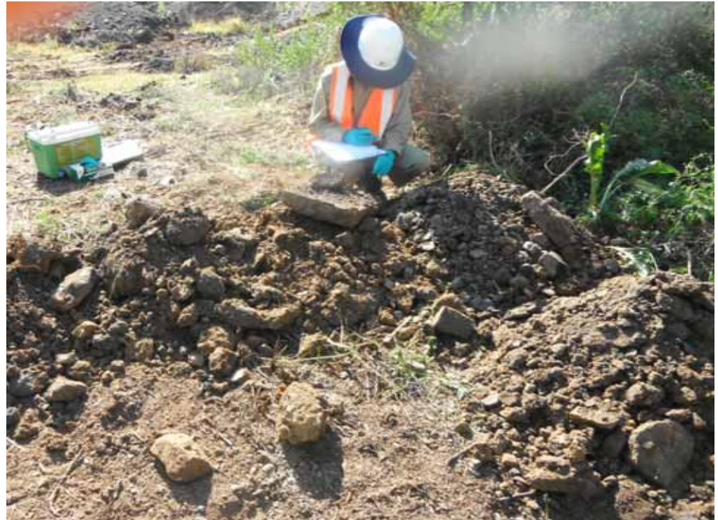
Test Pit 12 - Asbestos identified in soil sample
