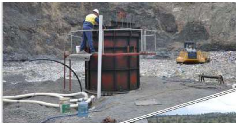
Figure 4: Central Leachate Riser
