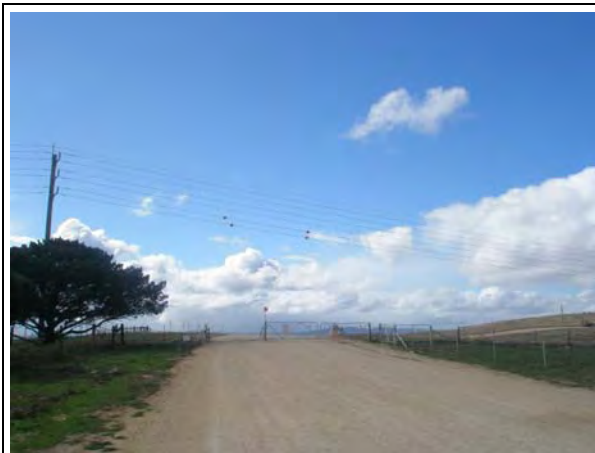
Plate 6.6 – Double circuit 33 kV overhead line crossing Capital Wind Farm access track
