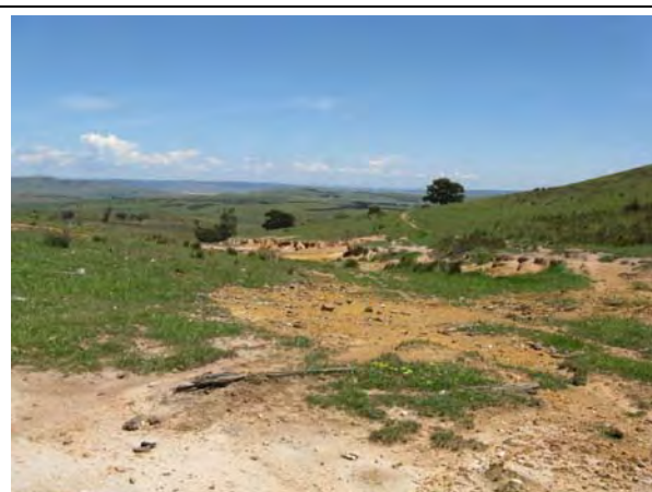
Plate 5.13 – Existing erosion between Turbine 11 and Turbine 12
