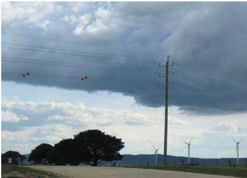
Plate 3.3 – Typical double circuit single pole 33 kV overhead transmission line
