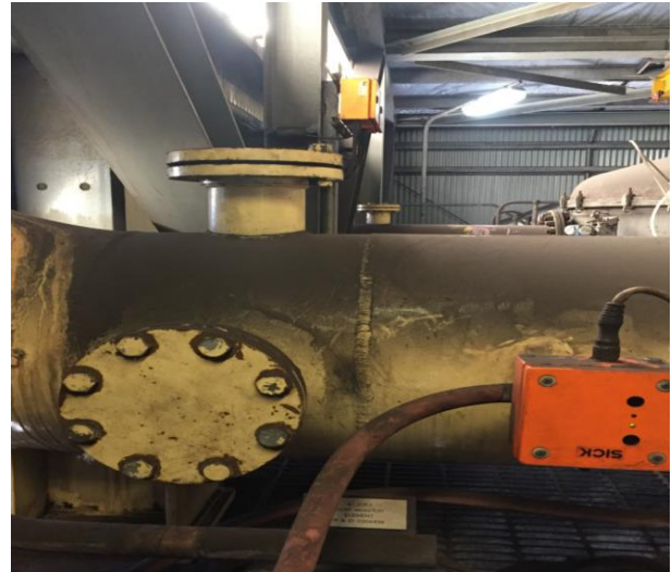
Figure 2 – EPA ID 106 - Depressurising Bag Filter Stack (West)
