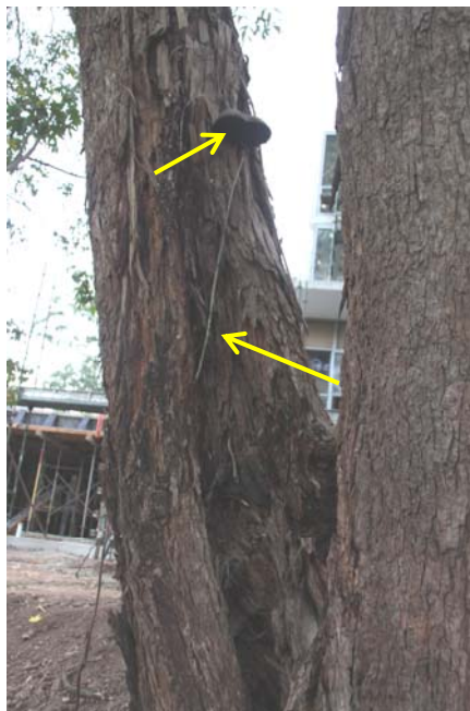
T49- Decay extends up the leader to three metres from ground to root crown. Fruiting body of Phellinus robustus at apex of decayed wood
