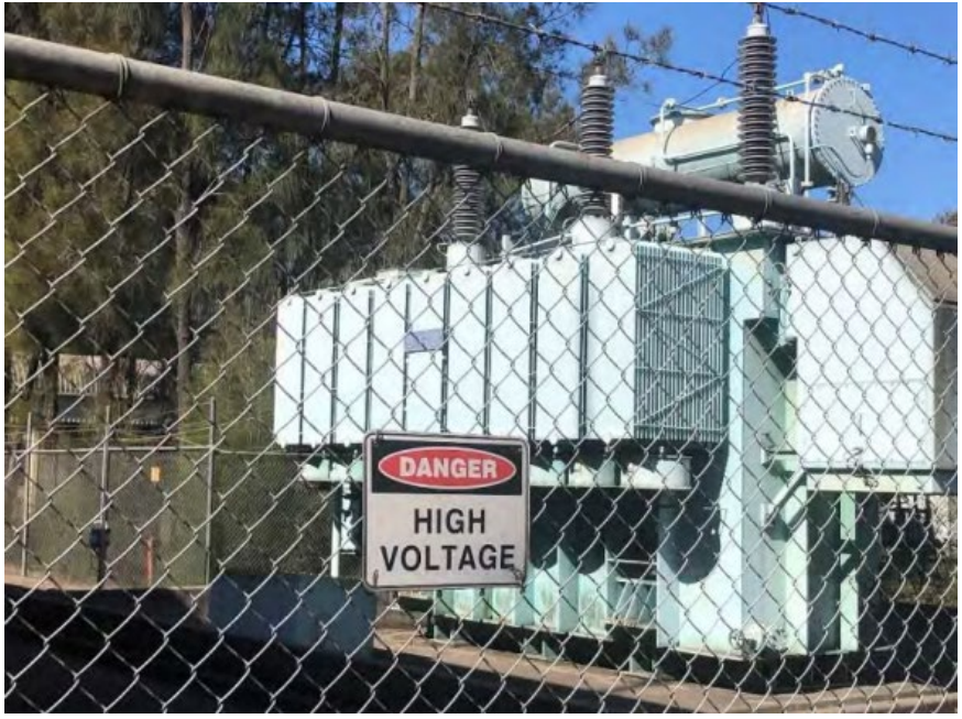
Figure 4 | Existing Transformer to be Moved
