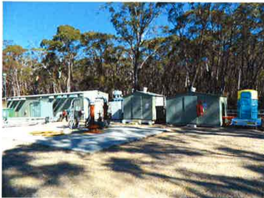
Photo 1 - Bore 6 Dewatering Facility
