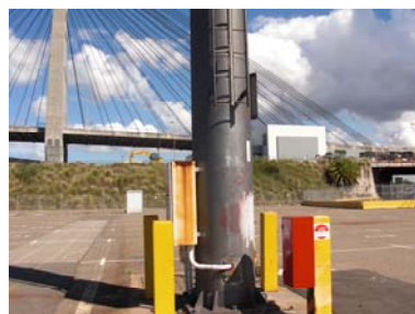
Lighting rig ladders
