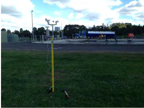
Weather Station installed to east of odour source
